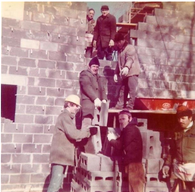
Paul Hoenisch and the rest of the volunteers handing up the cinder blocks to expand the building to what it is today
